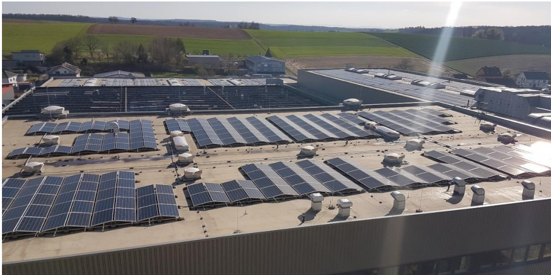
Figure 7: Photovoltaic system in Kirchartd Source: Picture taken by Friedrich Lösch (KACO)
