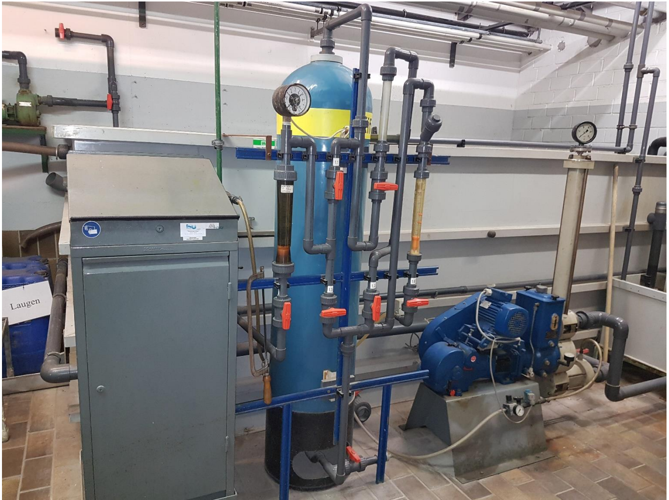
Figure 10: Waste water treatment
